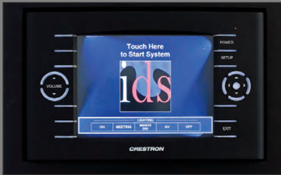
Crestron TPS-6X touchpanel wall mounted at IDS. The touchpanel releases from the docking station and used wirelessly anywhere in the room.
