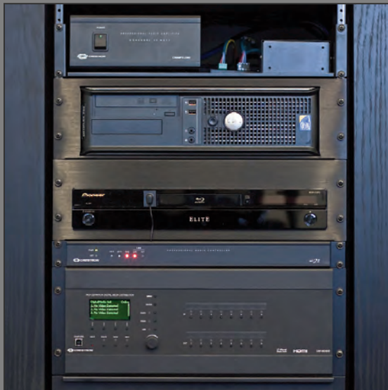
Equipment rack in the Presentation Room, with Crestron DM-MD8X8 DigitalMedia switcher, MC2E processor, CNAMPX-2X60 amplifier, plus Pioneer Elite Blu-ray player and Dell Optiplex computer installed.
